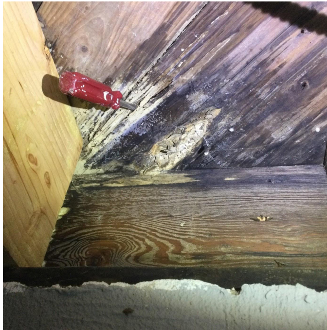
Mold and wood deterioration in basement floor structure.
