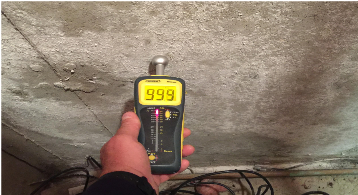
Elevated moisture meter reading on a foundation wall with efflorescence.
