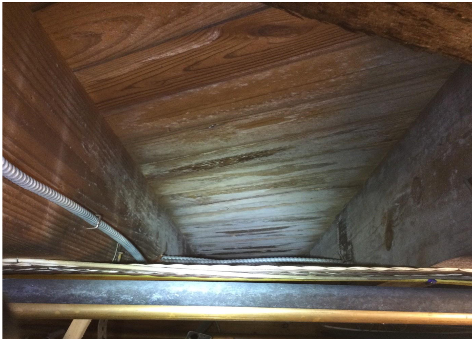
It is not uncommon to see this type of mold growth due to lack of proper dehumidification.
