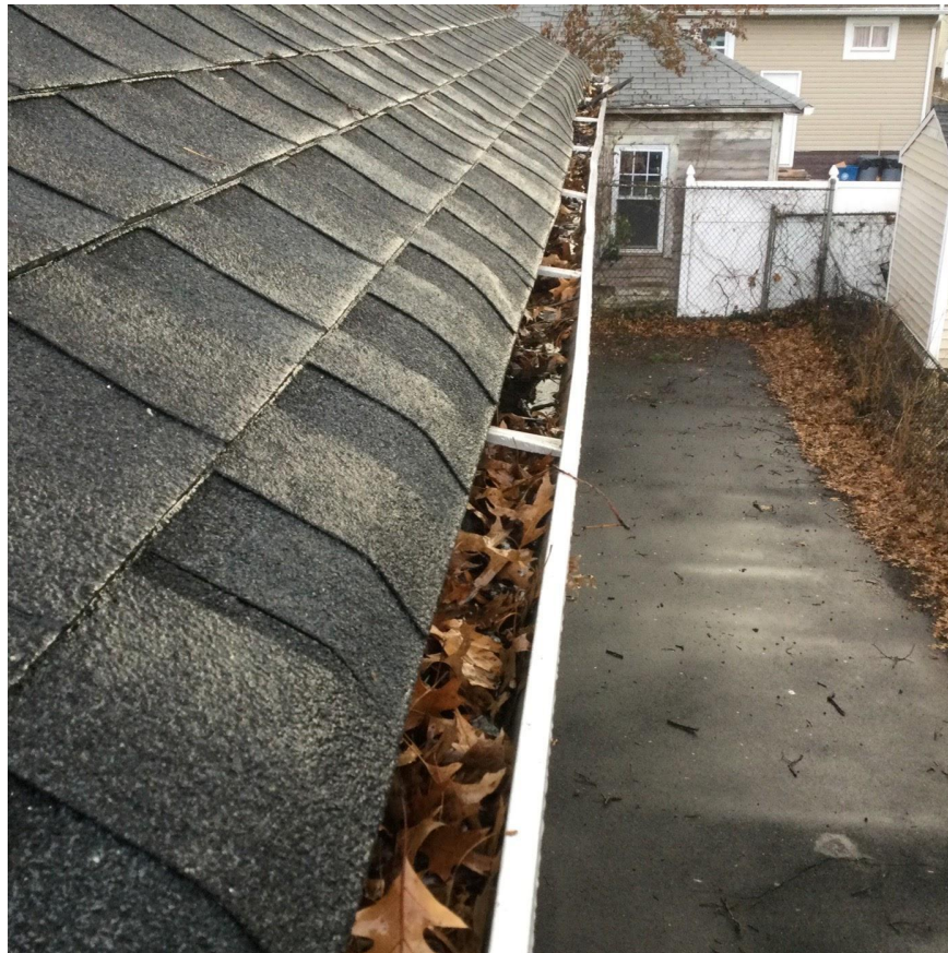
Clogged gutter system.
