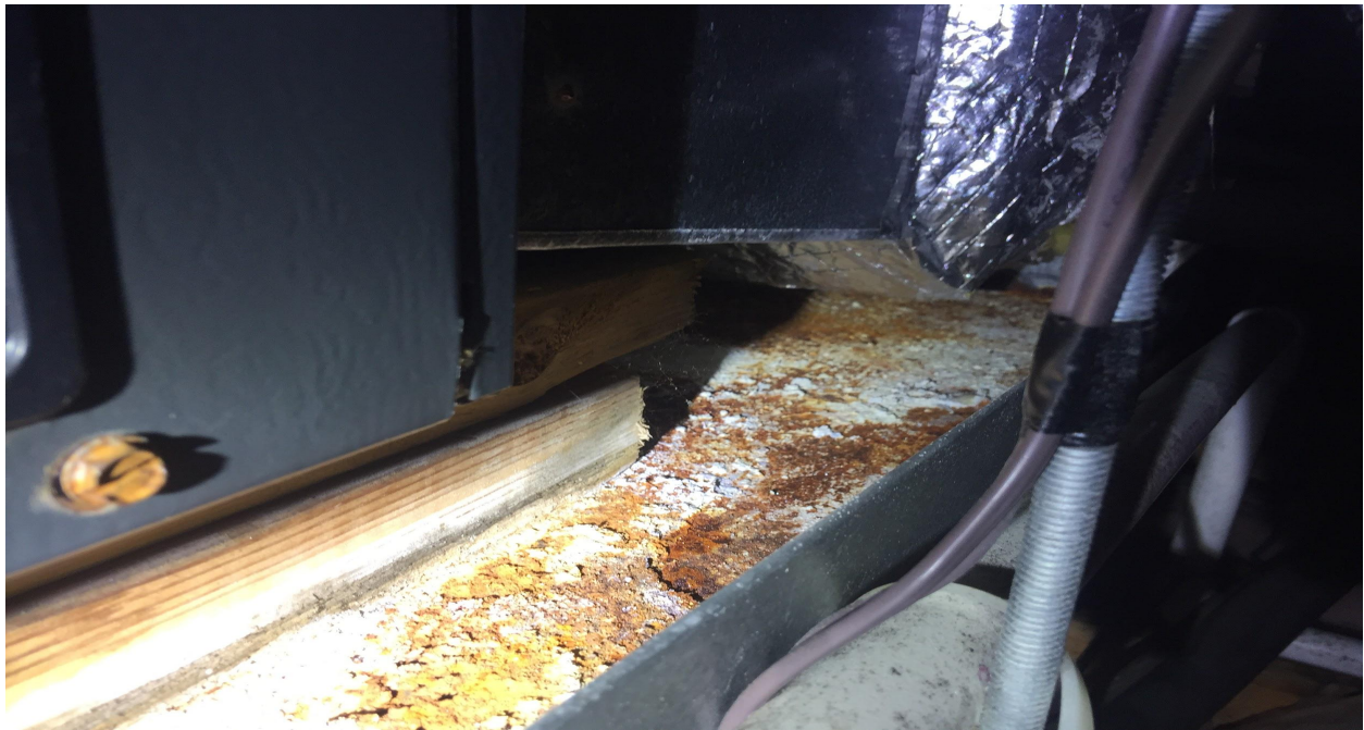
A defective evaporator coil in the attic can cause water damage leading to mold growth.
