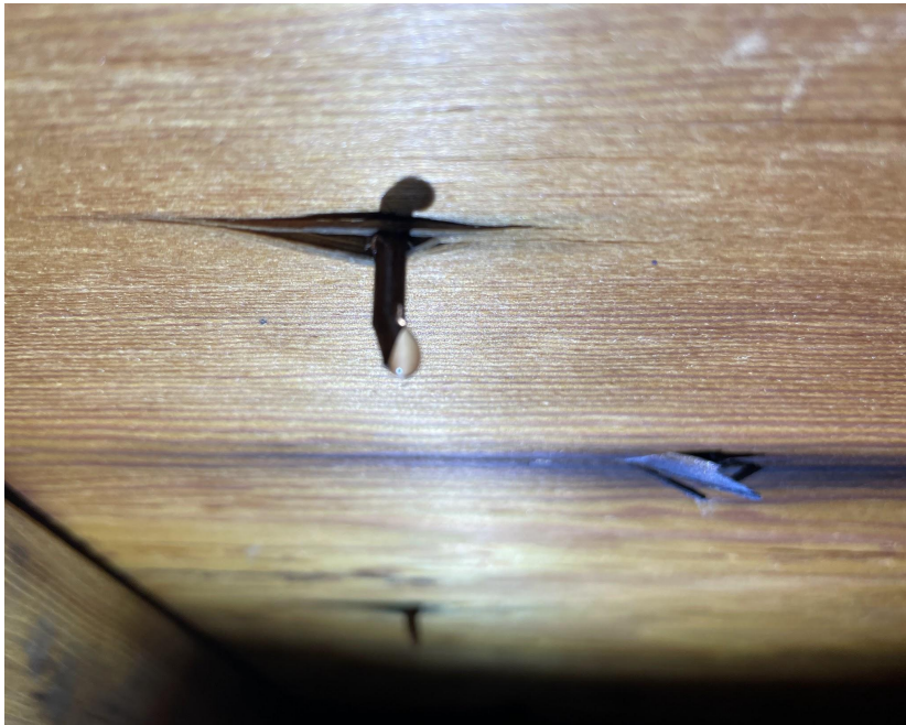
Condensation on nails in the attic can promote mold growth.
