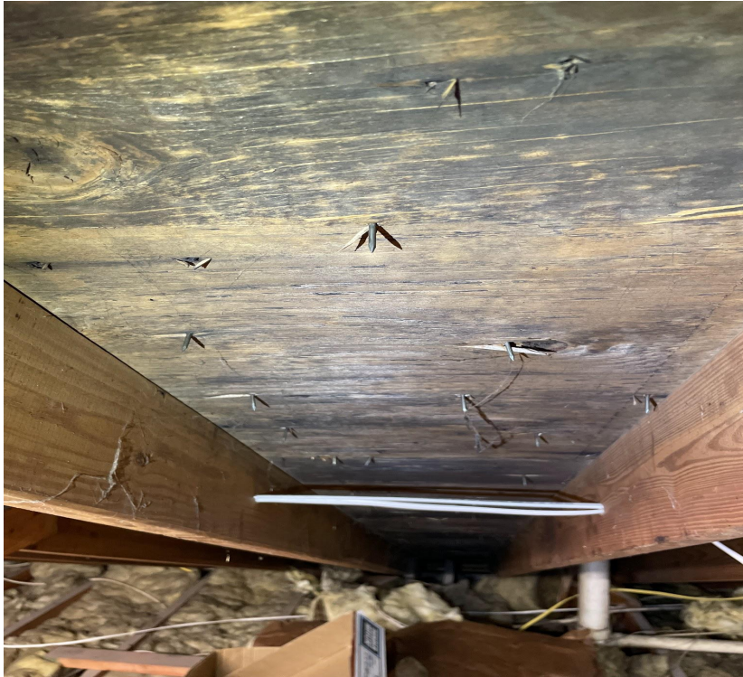
Mold on sheathing due to improper ventilation.
