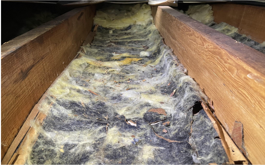
Rodents pushed insulation for nesting. This caused condensation and mold in the bedroom below.
