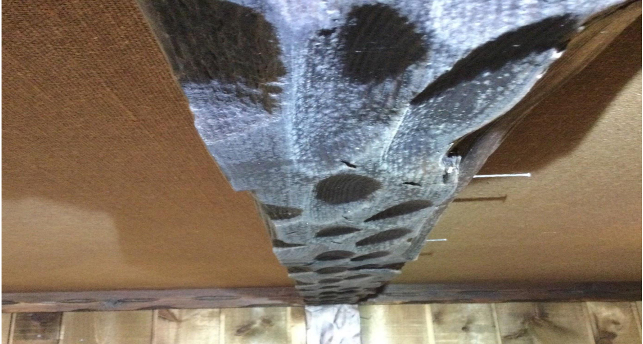
Mold on the basement ceiling due solely to lack of dehumidification.
