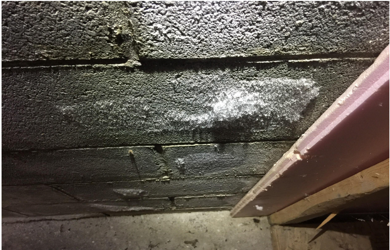
Mold can grow on organic substances embedded on concrete.
